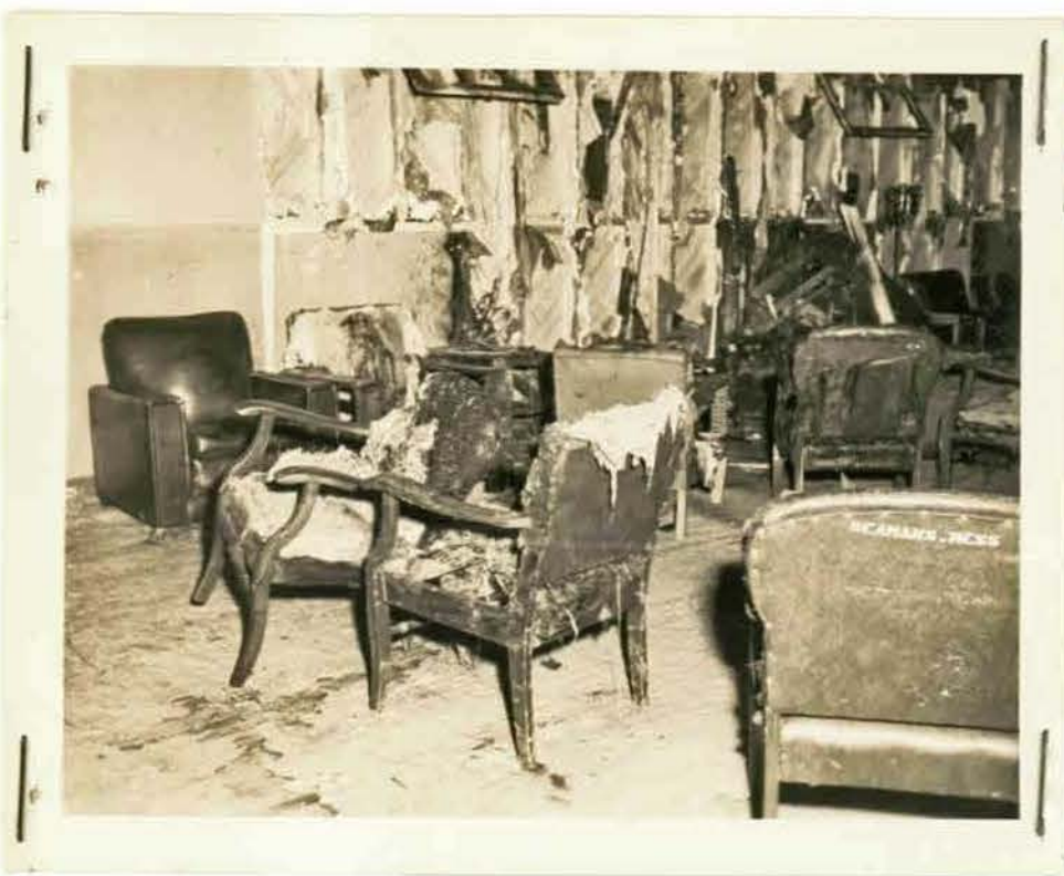
Neg. No DB 7744 Dispo: L HQ Dest Photo'g Manuel Dept FIRE HALL Caption SHIPS COMPANY MESS FIRE View of damage to the interior of the lounge.
