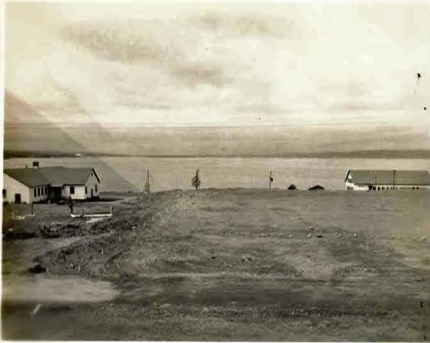
DB: 9231 DISP: L/HQ West. Photog: MANUEL Dept: Maintenance Progress photo of new Sports Field, looking west from Wardroom
