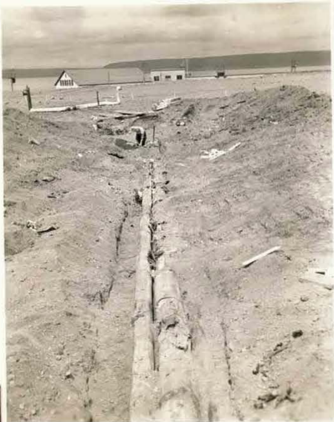
DB 9235 Dispo. L. ✓ HQ. Dest.. Photog. Manuel Dept. Maintenance Progress photo of New Sports field. Water line being taken out.
