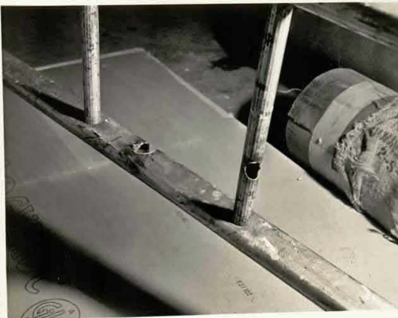
14770 L Porter Safety Office 30-12-60 Aluminum Ladder. Result after aluminum ladder was in contact with 220 V. electric wiring.
