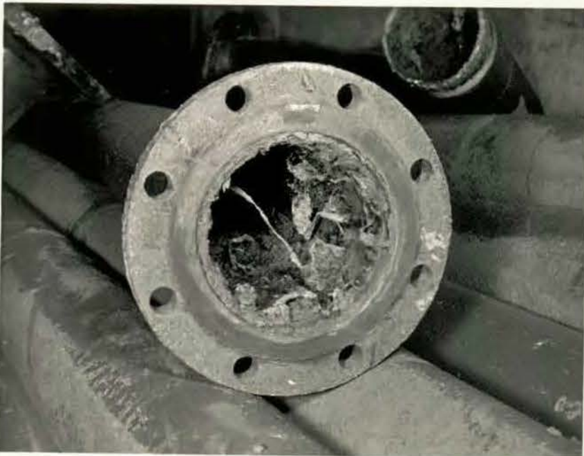
H.M.C.S. CORNWALLIS NEG. NO. DE. 19528 DISPO L x HQ D PHOTG. ESTENSEN DEPT. WORKS DEPT. DATE. 16-12-64 CAPTION..... PIPE CORROSION
