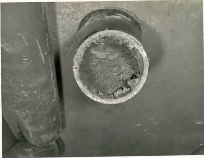
H.M.C.S. CORNWALLIS NEG. NO. DE. 19527 DISPO L x HQ D PHOTG. ESTENSEN DEPT. WORKS DEPT. DATE. 16-12-64 CAPTION..... PIPE CORROSION
