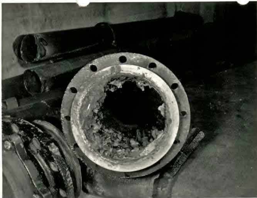
H. M. C. S. CORNWALLIS NEG. NO. DB. 19529..... DISPO L * HQ D PHOTCG. ESTENSEN..... DEPT. WORKS DEPT..... DATE. 16-12-64..... CAPTION..... PIPE CORROSION.....
